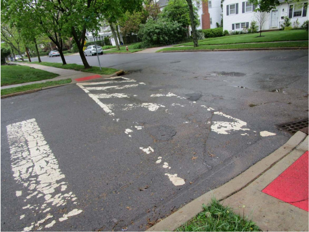
Figure 20 - Crosswalk wear, Lawrence Ave. at Madison Ave.
