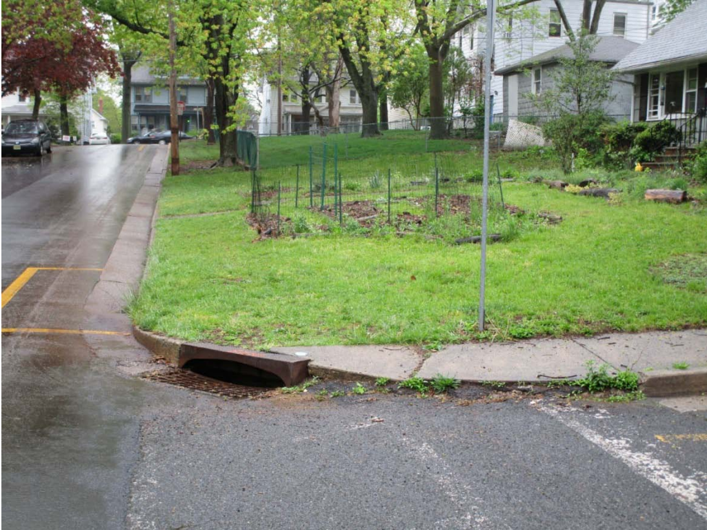
Figure 16 - Missing sidewalk and curb ramp, Mansfield St. at Braun Ave.
