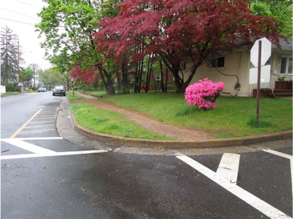
Figure 7 - Missing sidewalk and curb ramp with worn path, Central Ave. at Merlind Ave.
