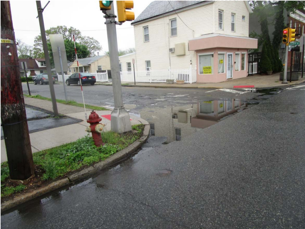
Figure 12 - Drainage issue, Woodbridge Ave. at S. 11th Ave.
