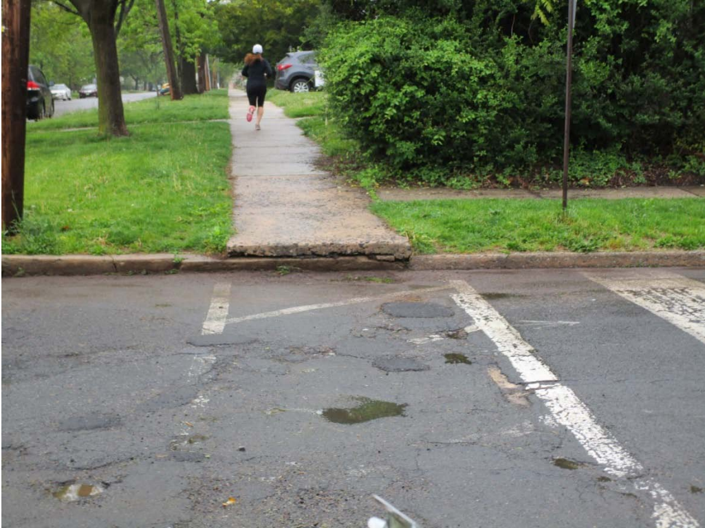
Figure 15 - Missing curb ramp and worn crosswalk, Harper Pl. at S. 3rd Ave.
