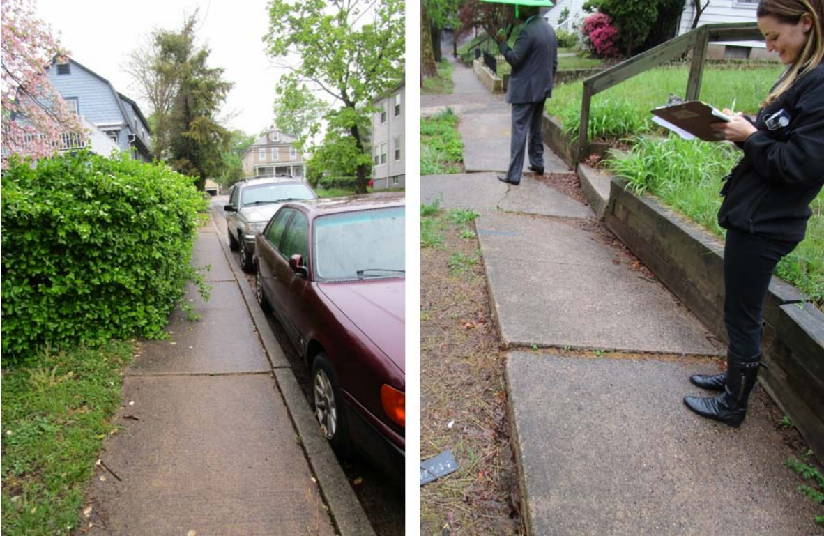
Figure 17 - Examples of vegetation encroachment and sidewalk uplift in the Bartle neighborhood
