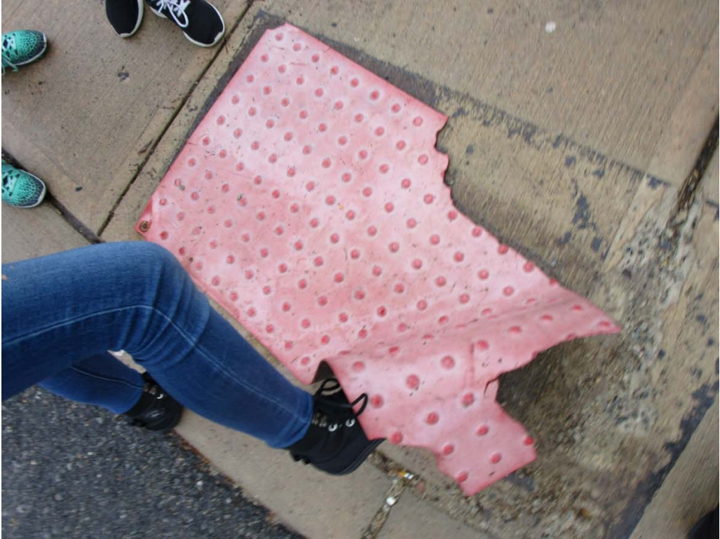
Figure 19 - Truncated dome pad in disrepair at Middle School entrance
