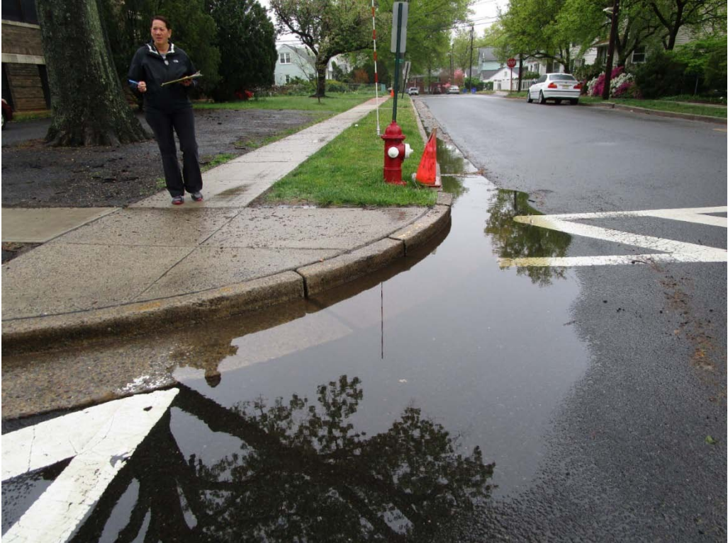
Figure 9 - Drainage issue, Central Ave. at Merlind Ave.
